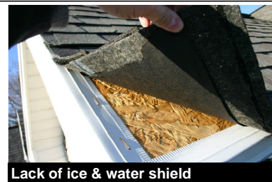
Lack of ice & water shield
