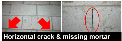
Horizontal crack & missing mortar
